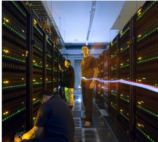
Figure 1-1 Weta Digital Data Center
